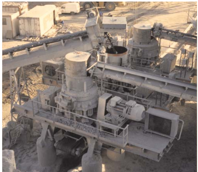
Plant with DUSTEX® in operation
